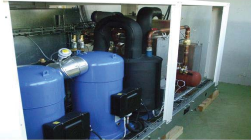
Figure 6-11: Picture of the Altereco heat pump
