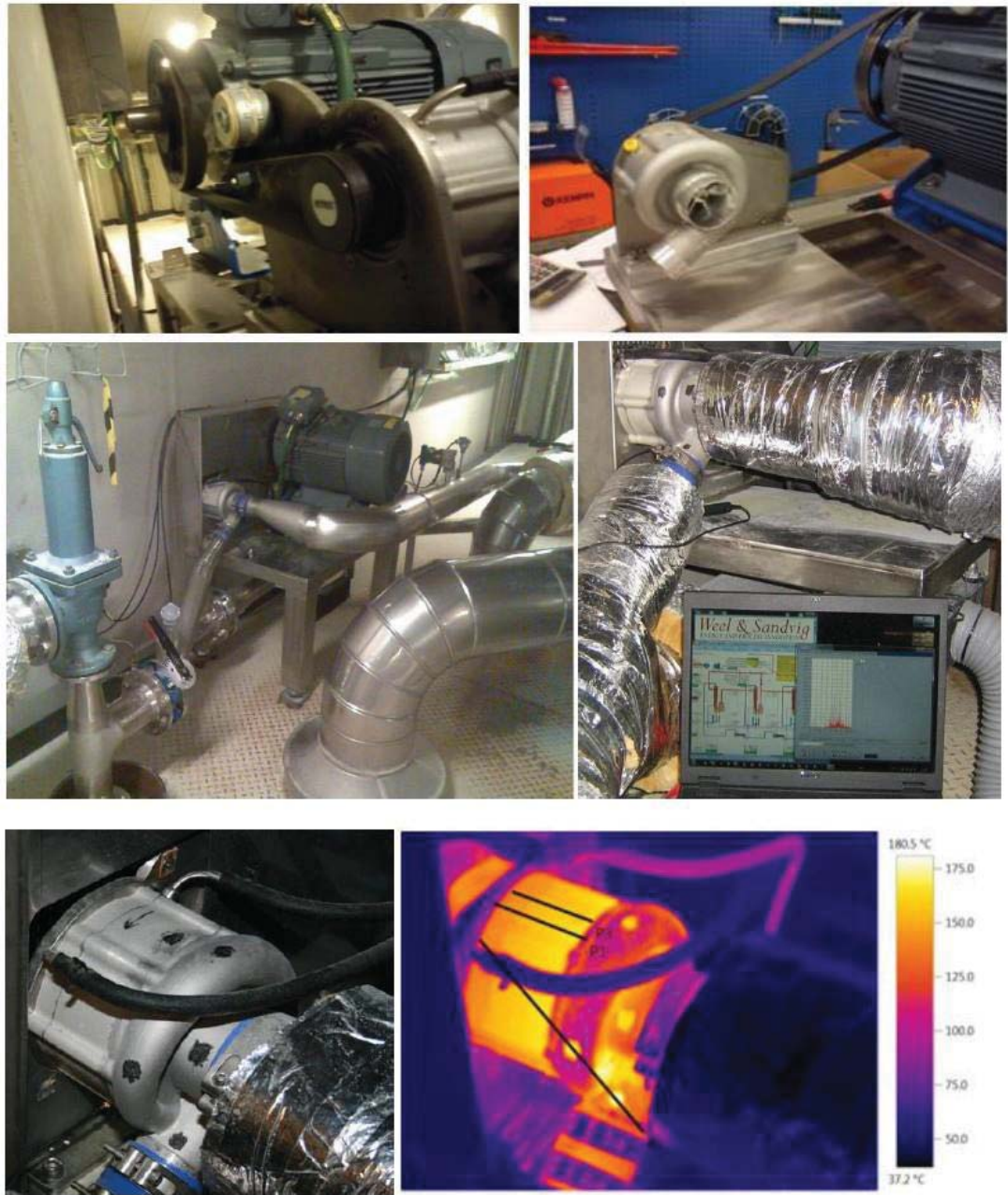
Figure 5-10: Pictures from the first heat pump test at Haldor Topsøe's production facility in Frederikssund, Denmark
